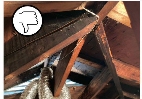
Example of Hip Cracking from Age
