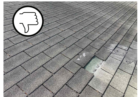
Example of Missing Shingles
