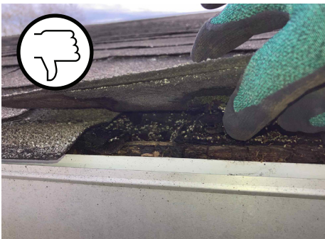
Example of Rot at Decking
