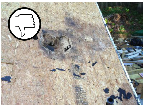
Dry rot or other damage
