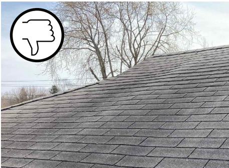
Example of Visual Sagging on Roof
